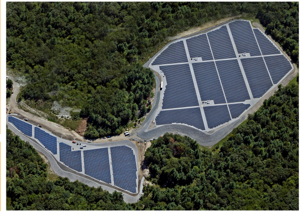
Project: Westford Solar Field • Location: Westford, MA System Size: 4MW • Installer: NexAmp • Product: SGI 500
