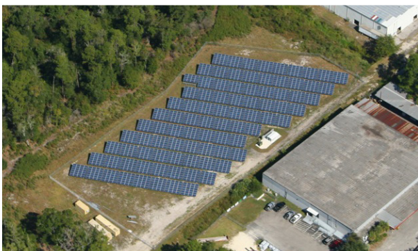
Project: Gainesville Solar Farm • Location: Gainesville, FL System Size: 5MW • Installer: Sybac Solar • Product: (10) SGI 500
