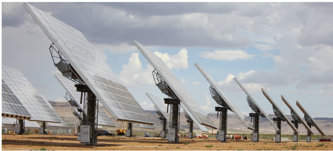
Project: XCEL Energy Solar Farm • Location: Alamosa, CO • System Size: 30MW • Installer: Amonix Product: (504) PVI 82KW, SCADA Controlled & VAR Support
