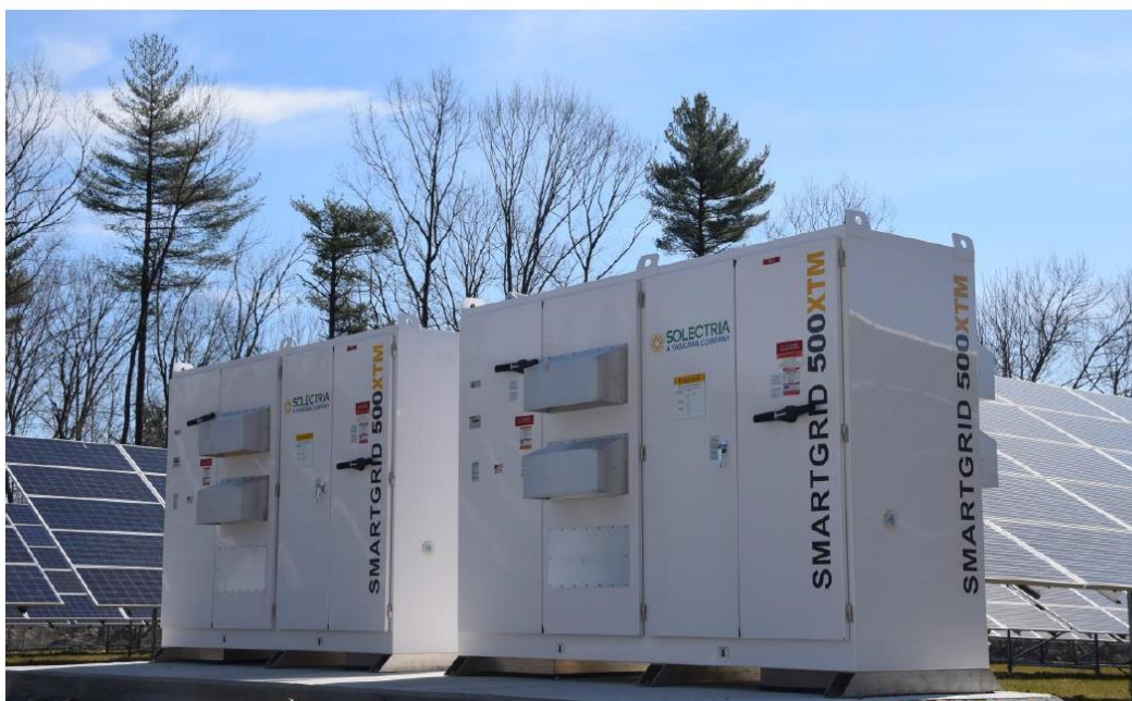
Figure 14. 1.0MW PV plant with grid supporting functions in Shirley, MA
