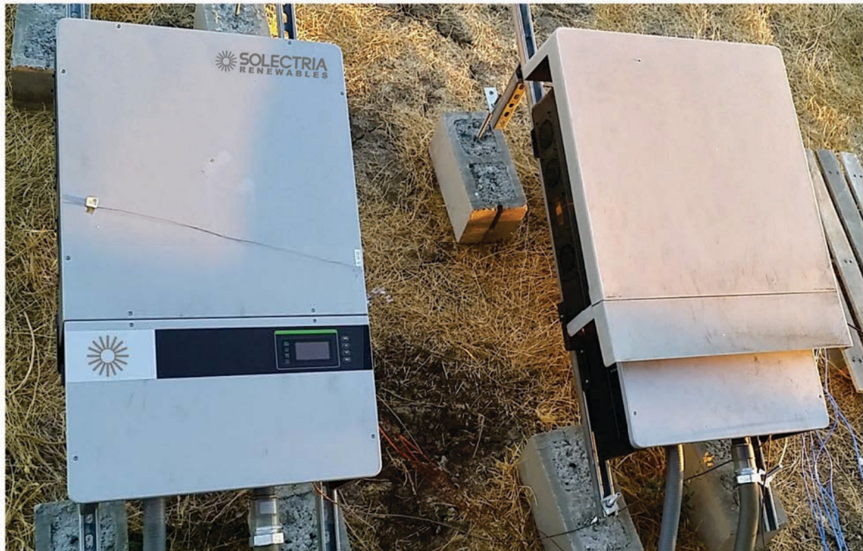
Figure 2 Image of the installations of the two (2) Solectria PVI 28TL – the inverter on the right-hand side of the image has a shade cover installed
